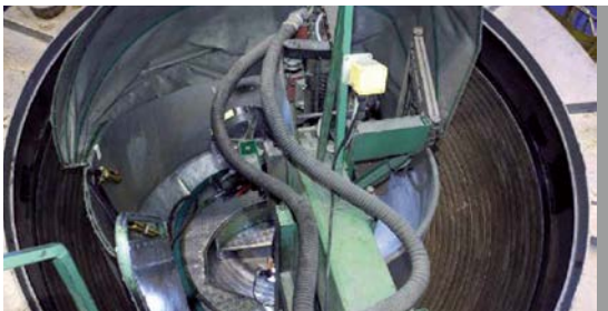
Steam Generator Expansion Tank Soudotape 308 L Q5 + Record 8B308T1 Q5 Soudotape 309 L Q5 + Record 8B308T1 Q5
